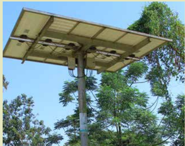
Solar powered water pump panel
